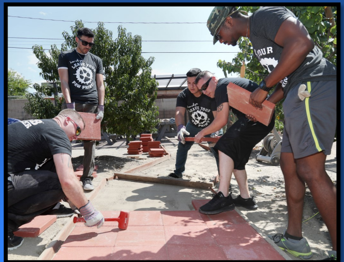
CSUSB staff and students assemble a brick walkway at the DAV Garden.
